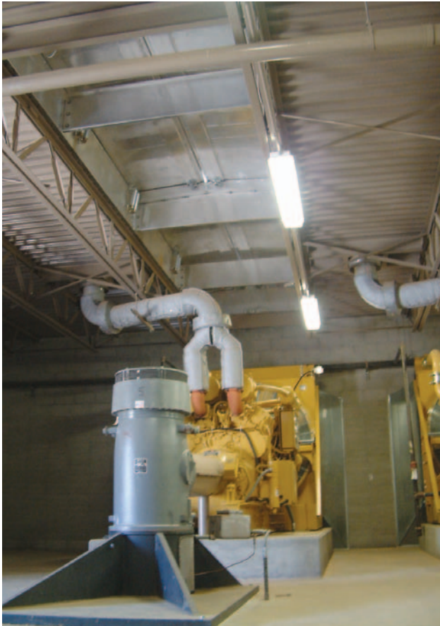
The above-ground portion of an ADOT pump station has ports in the roof to allow the engine/pump packages to be lowered into place with a crane. The stations also have to be located near natural gas lines to fuel the engines, near sources of runoff water, and near a river, canal or open desert area that can accept the discharge water.
